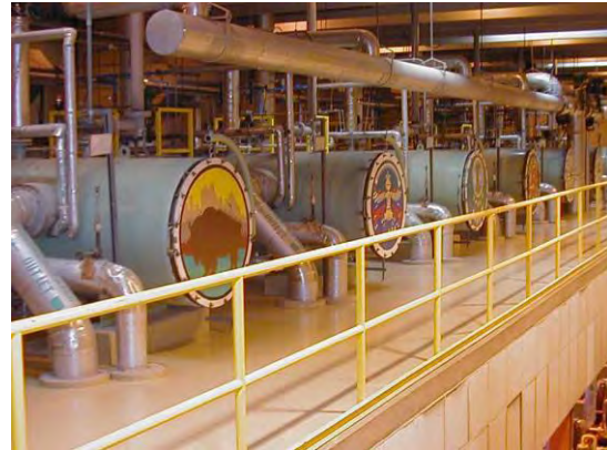
Boilers, located above the engines
