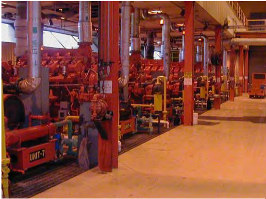
Seven 650-kW Waukesha engines
